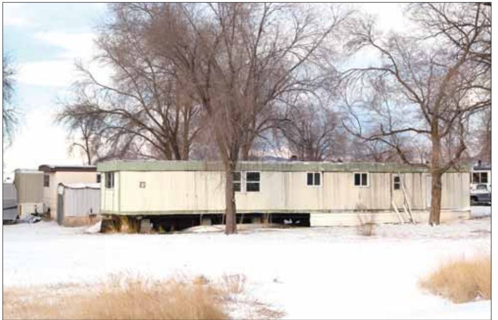
TRAILER PARK PROBLEMS • The Levan City Council wants to see progress in fixing up this trailer park in Levan.
